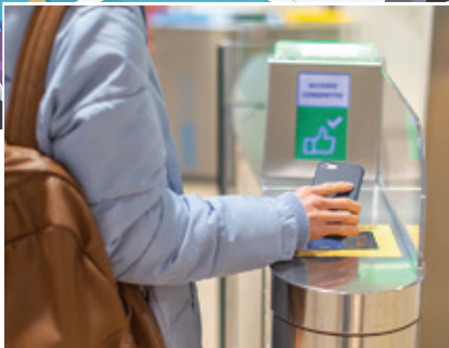
Turnstile Access Control, Entrance Security Railing Gate System
