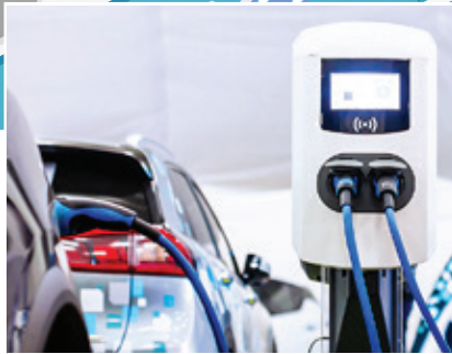
Electric Vehicle Charging Station HMI Control Interface
